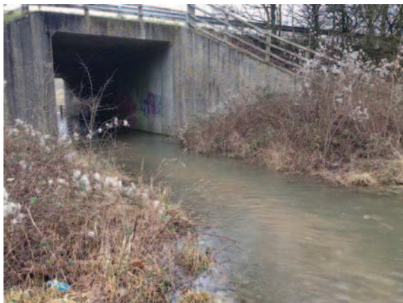
Figure 7: Flooding at public footpath east of a339 near Vodafone surface water runoff 350mm
